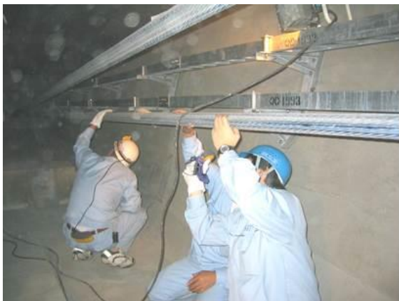
ECS inspection in box girder at BY433 Bridge, Japan after 10 years' service. No abnormality found.
