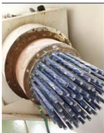
ECS stay cable and anchorage inspection after about 30 years' service. No abnormality found.
